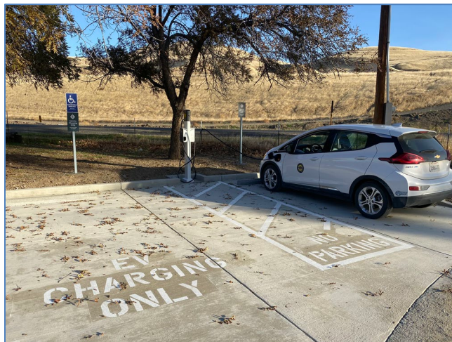
Figure 2-17: EV Charger installed in 2022 near the Carnegie SVRA Ranger Station
