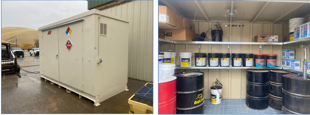
Figure 2-16: New Oil Containment System at the Carnegie SVRA Maintenance Shop
